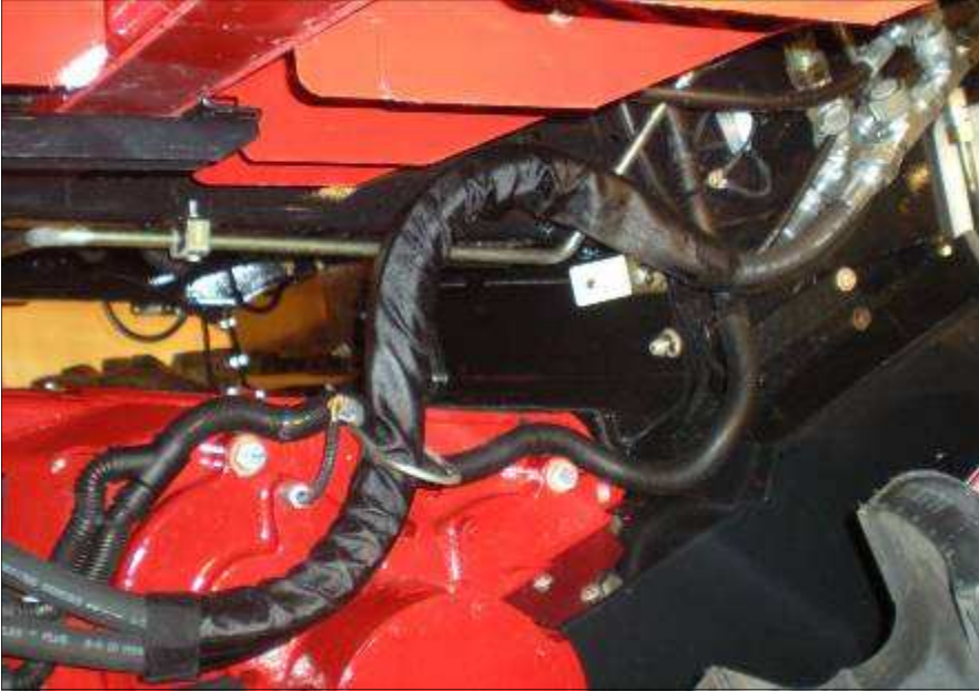
Custom sleeve installed by CNH to bundle and route the hydraulic hoses
