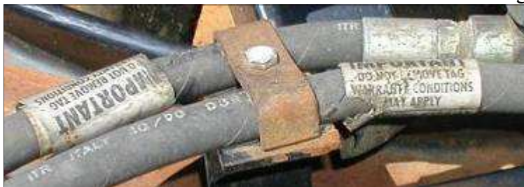
Judging by the label, they must have figured the clamp would lead to failure (under warranty). 1 Notice how the cover and sticker have been gouged by the clamp.
